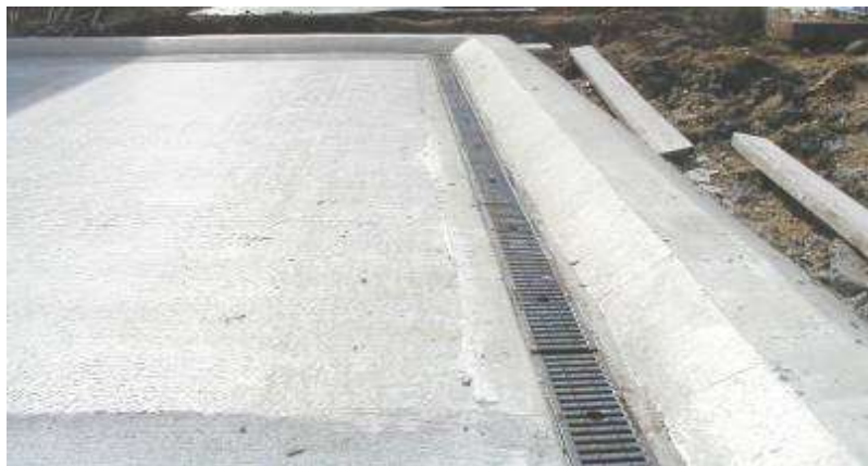
Concrete pesticide handling area with bund and ACO type drainage system
