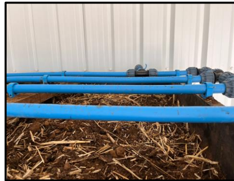
Proprietary Biofilter pipework
