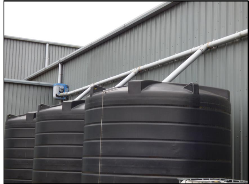
Rainwater collection systems increasingly being fitted to sprayer centre developments.
